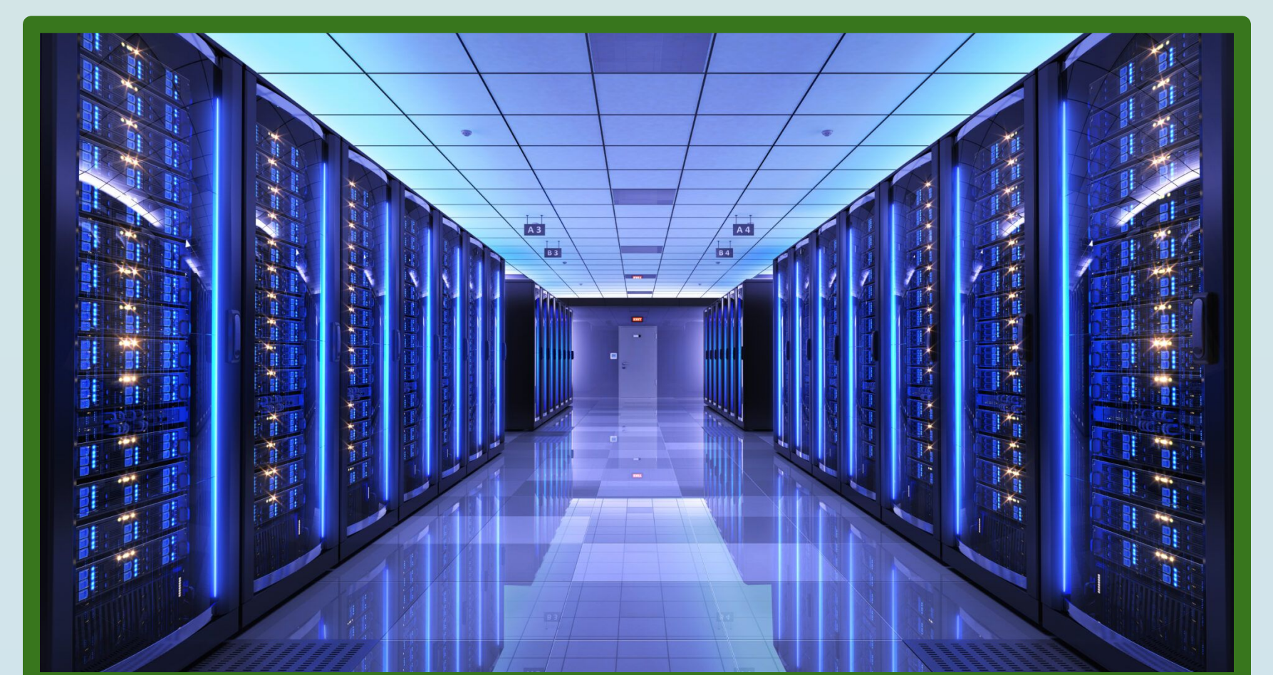
TRG Data Centers; a major data center operator, based in Houston ( https://www.trgdatacenters.com/resource/what-are-data-center-solutions/ )
