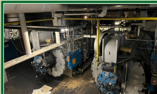
One of three boiler rooms on campus
