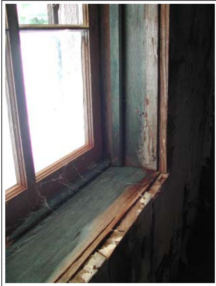
Figure 4.13. Light blue paint on interior window trim of the A. Ilseng House, Bosque County, Texas.
