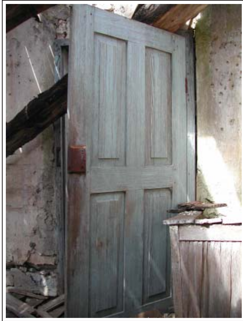
Figure 4.12. Light blue paint on interior door of the Jens and Kari Ringness House, Bosque County, Texas.
